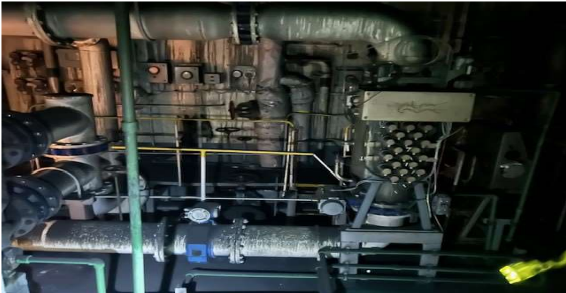
Figure 15- Oil streaked down the forward bulkhead in the engine room on two decks. Images taken on January 11, 2024 by the U.S. Coast Guard.
