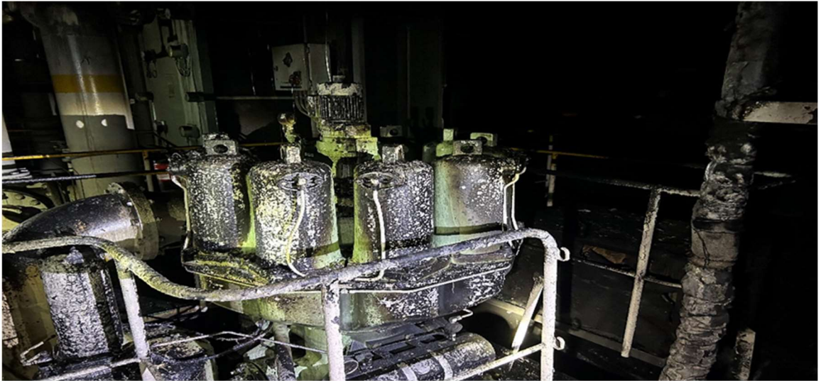
Figure 12: Lube oil filtration system located within the high-temperature exposure area. Images taken on January 11, 2024, by U.S. Coast Guard.
